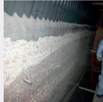
Abrasion in a combustion chamber
