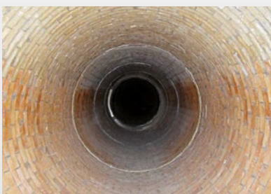
Tertiary air duct. Lined with fireclay bricks.
